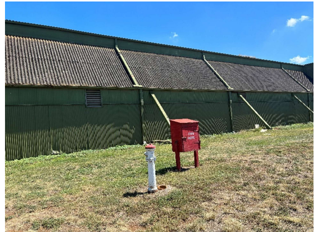
The far side of our restoration hangar after the area was cleared, the wall cleaned and repainted
